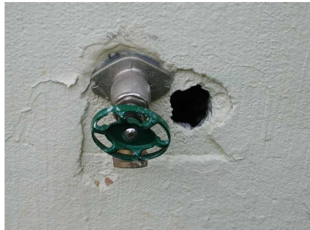
Figure 3. Holes in the foundation and around plumbing, conduit and wires should be sealed to prevent pest entry.
