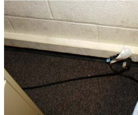
Bed bugs can move along wires and inside conduits such as they wall-mounted units.
